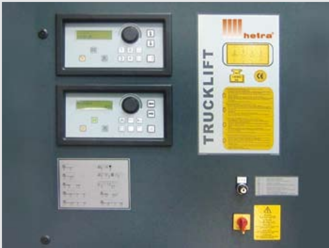
Central control and programming unit with two displays.
