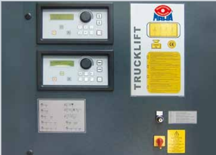
Central control and programming unit with two displays.
